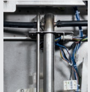
Stainless steel ascending pipes
